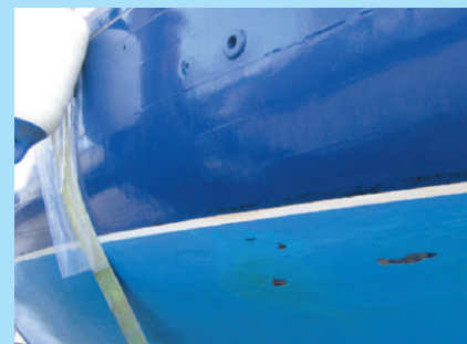
Here the paint finish is good, but has cracked and raised on the seams
